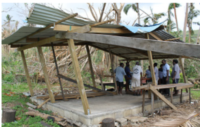
The Emua Market House was completely destroyed after Cyclone Pam in March 2015. Photo: Ellie van Baaren/UN Women.
